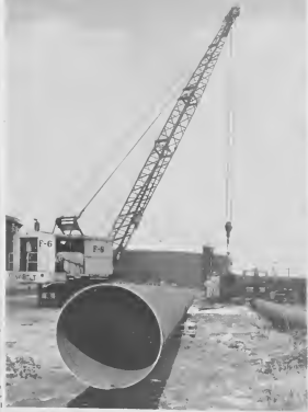
FROM THIS angle the 36-inch pipe looks even bigger. It will be able to handle 30,000 barrels an hour.
